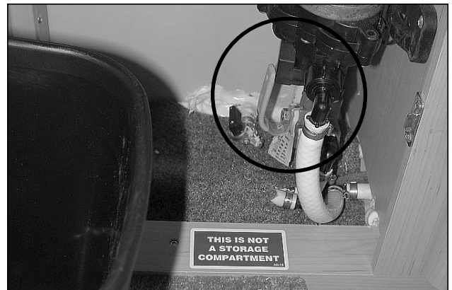
Picture G-P2: Selector valve position for supply from the exterior fresh water tank.
